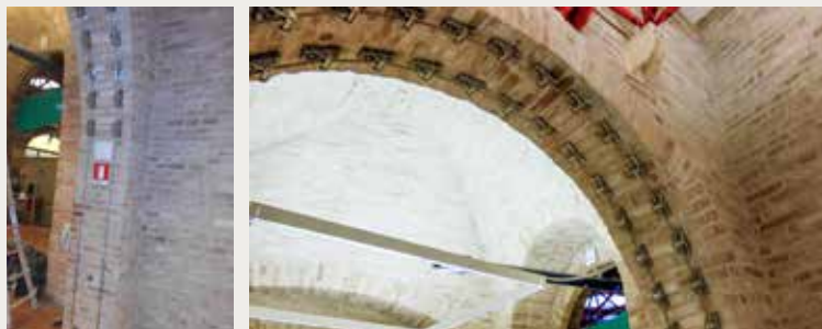
Reinforcement of one of the arches on the ground floor, the reinforced arch technique opposes the formation of the hinges, which open alternately to the intrados and extrados, positioning a cable stretched across the intrados of the arch or vault.
